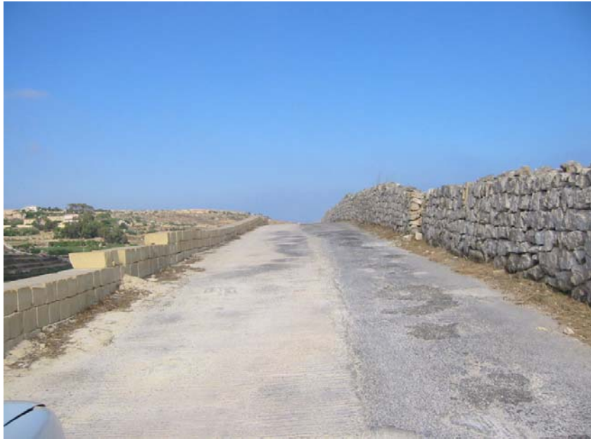
Photo 7: Boundary walls (to the left) along Triq Ta' Gruwa panoramic road need to be replaced by aesthetically acceptable rubble walls
