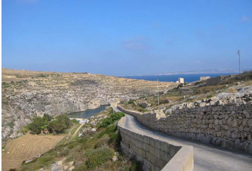
Photo 11: Boundary walls (to the left) along Triq Ta' Gruwa panoramic road need to be replaced by aesthetically acceptable rubble walls
