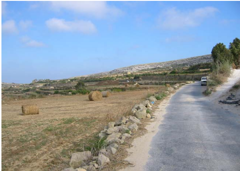
Photo 4: Collapsed walls along Triq Ta' Gruwa panoramic road conspicuously mar overall aesthetics
